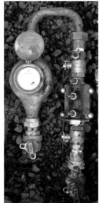
Typical double check valve assembly in box with meter (DCVA on the right).
